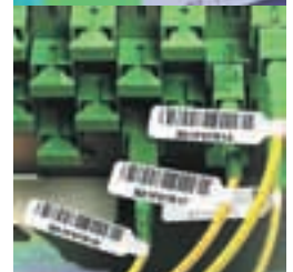
Fibre optic marking
